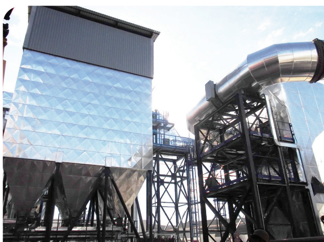
This plant ordered DID, MAS and SCR systems in order to ensure compliance with all future regulations.
