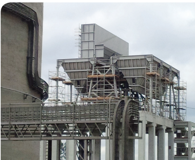
Installation took about half the time and much less space on site.
