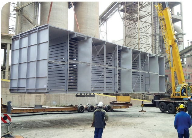
All 14 modules were pre-assembled with tailor-made lifting lugs installed in-factory for easy installation.
